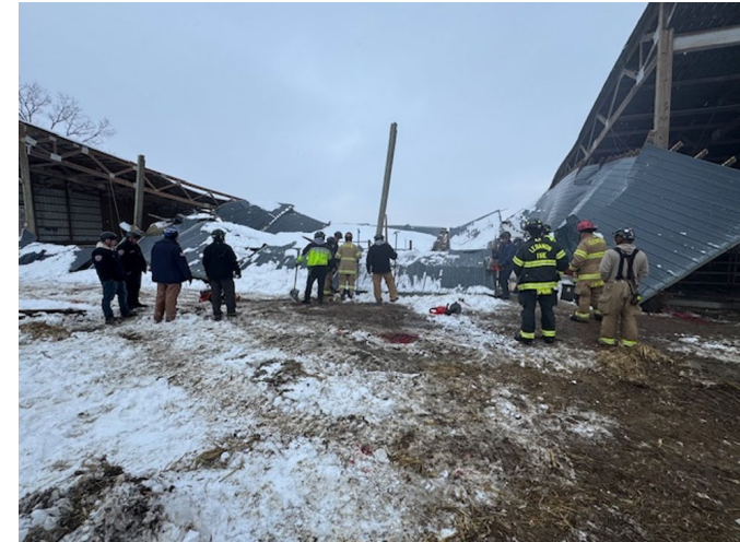
( Barn Collapse Waynesville )
